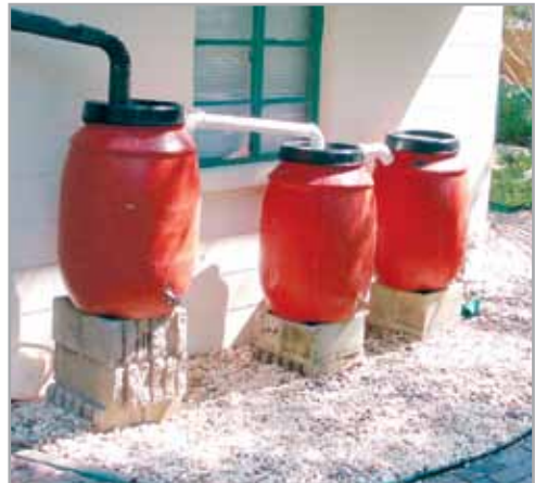
Multiple barrels provide for greater water storage.
