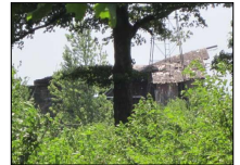
Example of Dilapidated structures within the Project Area
