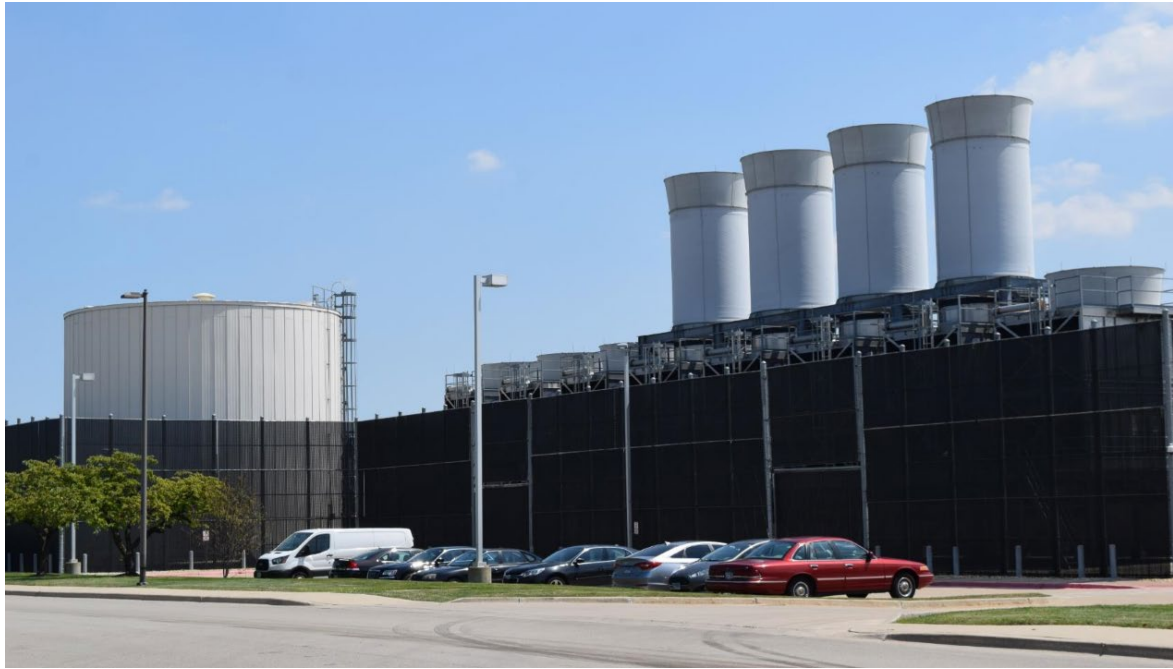
Water storage and cooling equipment, Digital Realty, Elk Grove Village, IL
