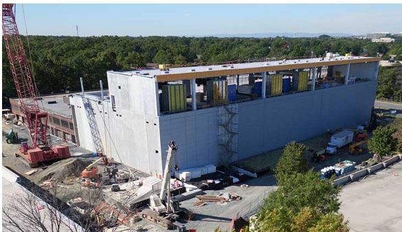
6 story data center, Coresite, Ashburn, VA
