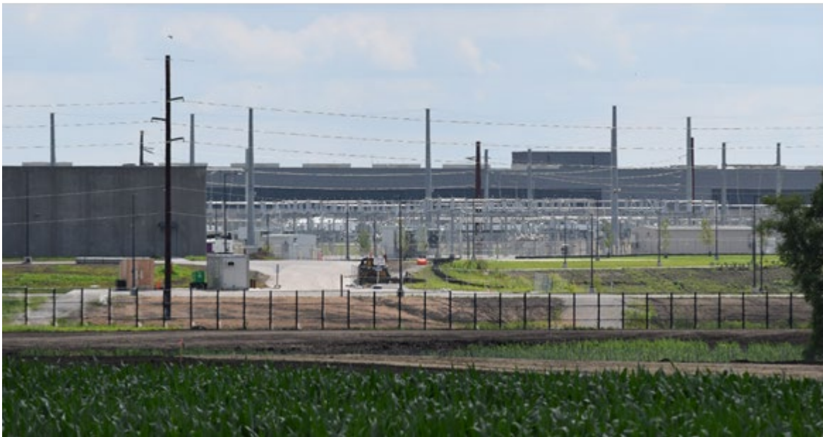
On-site electric substation, Facebook data center campus, Altoona, IA
