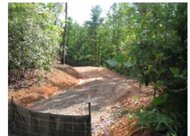
This is an example of a minor roadway under construction. This particular road will lead to a future residential subdivision development.
