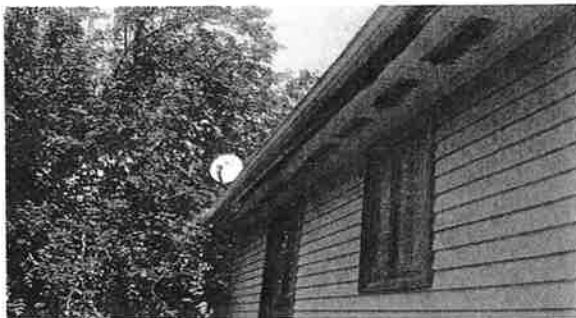
Possible animal intrusions at rear soffits (SEP, 06/06/13)
