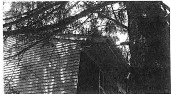
Possible animal intrusion at front soffit (SEP, 06/06/13)
