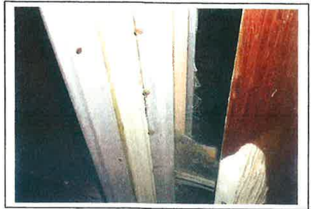
9/4/12 Broken windows TS
