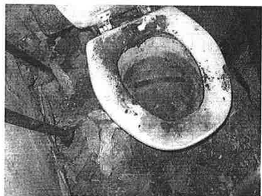
Fecal material in toilet (9/23/2009, LKJ)
