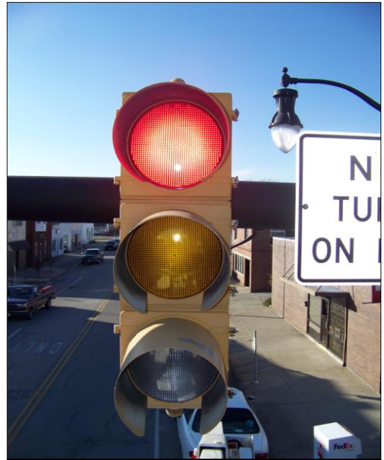
LED Traffic Signal Heads Installed in 2010
