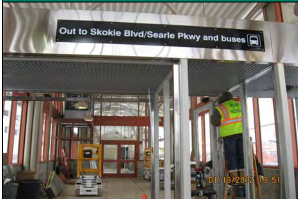
Finish materials being installed at the fare array at the North Station House
