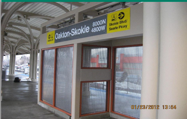
Windbreak frame and glazing on platform
