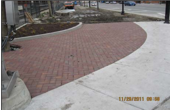
Decorative pavers and new concrete sidewalk at northwest corner of Oakton St./Skokie Blvd.
