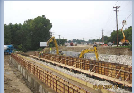
Pouring concrete for Pier Cap - Part of Bridge Replacement Over Rush Creek.
