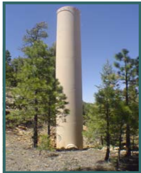
C. C. Cragin Surge Tank—absorbs variable pressure in the pipeline on its descent from the Reservoir.
