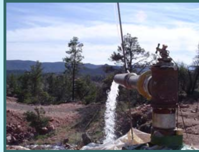
Groundwater being pumped from a TOP Well
